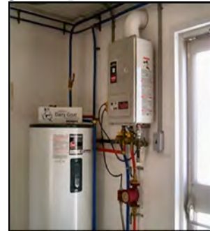
Fig. 21 Hot water tank in good repair
