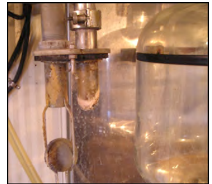
Fig. 47 Check sanitary trap for cleanliness
